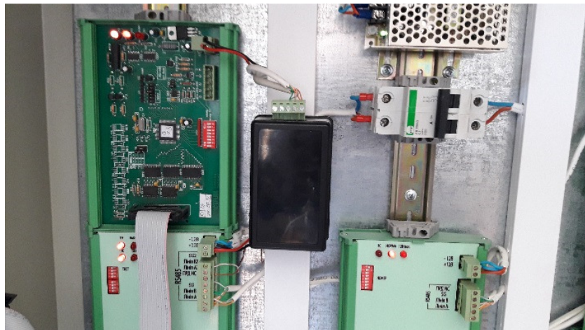
Figure 3. Connection of the receiver in the control cabinet via the RS-485 interface
