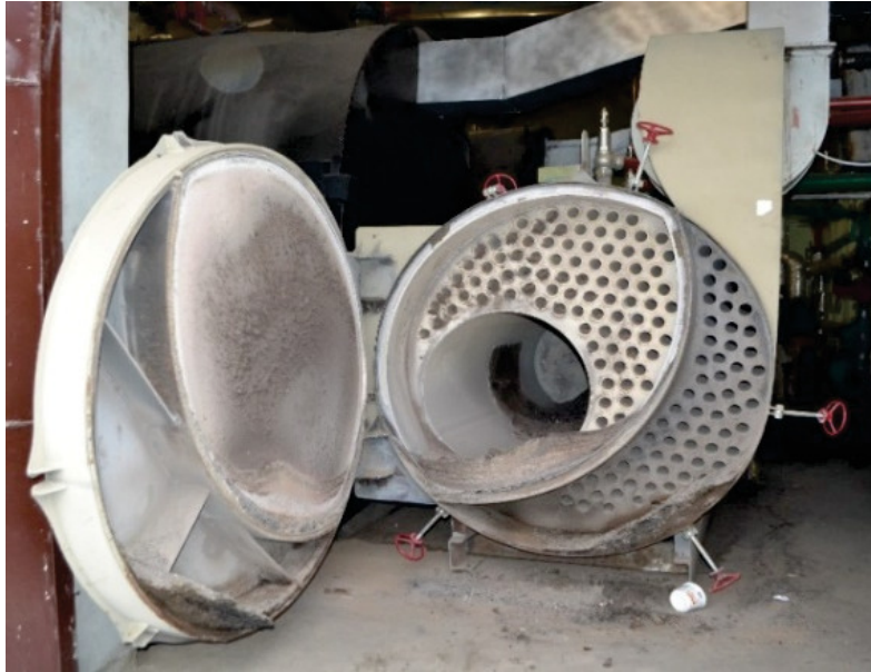
Figure 3. The final implementation of an industrial boiler with a capacity of 1 MW
