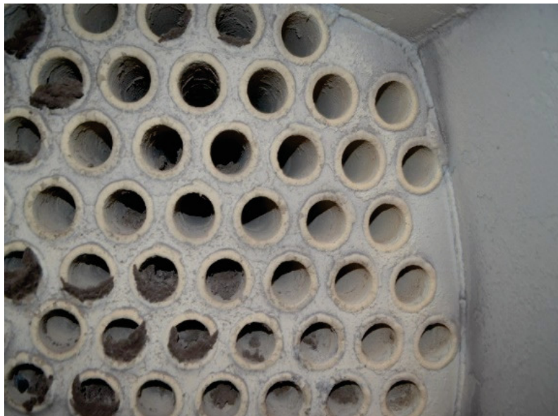
Figure 4. Photo of boilers heat exchanger surface in process of operations. No carbonization of firetubes and the white color of the ash on the heat exchanger surface testifies to full and clean fuel burning.
